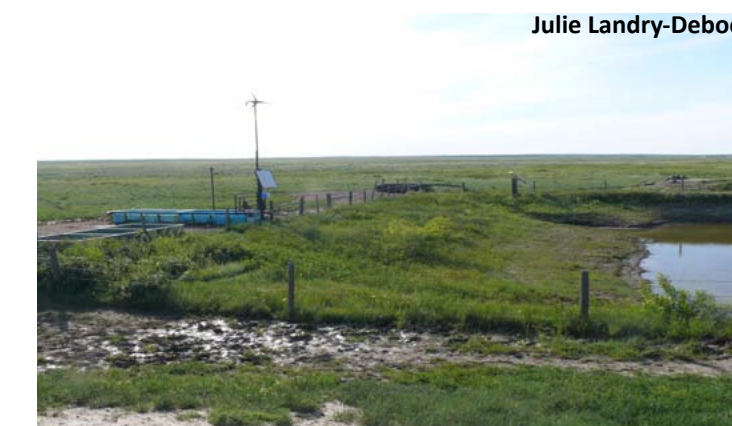
Fenced off dugout with various troughs using solar and wind energy to power pumps.
